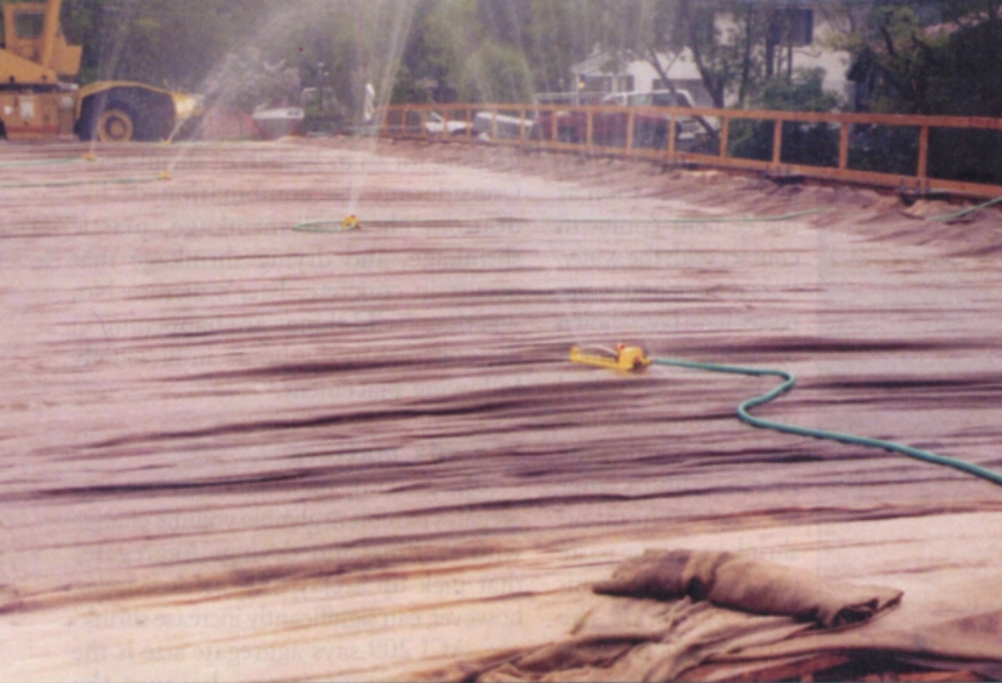
Facing page: Fog spraying increases the humidity of the air above the concrete and slows the rate of evaporation at the concrete surface. Above: Application of a full wet cure with burlap and soaker hoses prevents drying until the concrete is strong enough to be able to resist shrinkage stresses.
